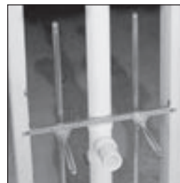
Test-ready stub outs and air chambers, with only ONE solder joint needed.
